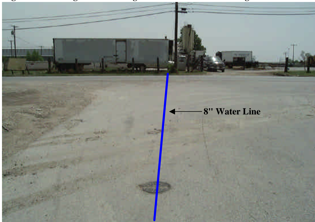
Figure 4 – Looking east at the water line valve near the corner of Fitchburg Street and Chalk Hill Road
