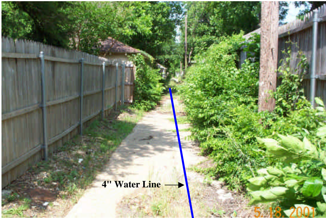
Figure 6 – Looking west from alley between Martel Avenue and Longview Street. Note: No wastewater line beyond this point.
